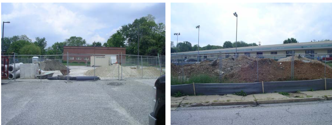
Figure 4-34: Uncovered Gravel, Dirt, and Other Construction Materials at ISI-A-924 Can Have Significant Effects on Water Quality During a Runoff Event. At This Location, Some Piles Were Properly Surrounded by Silt Fences but Others Were Left Uncontrolled.
