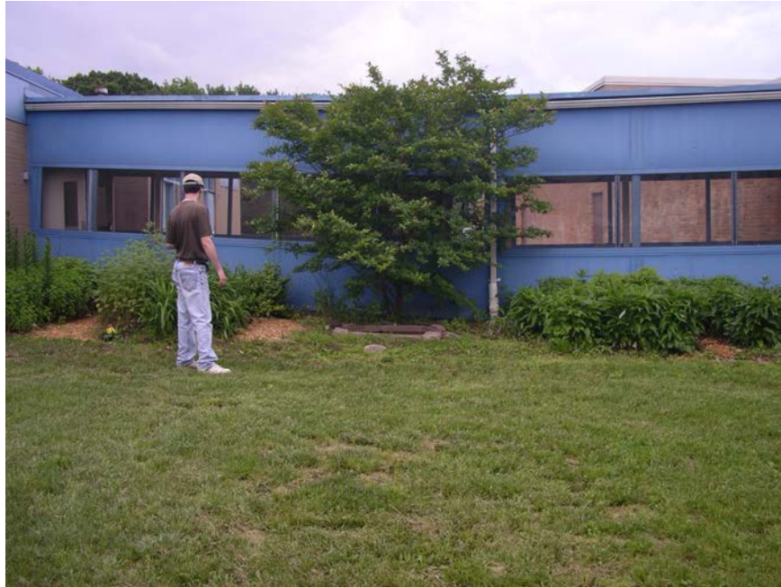
Figure 4-44: Staff at Relay Elementary School Complained of Flooding that Occurs at the Low Spot of this Breezeway. A Connected Downspout is Present Here and May be Redirected to a Newly Installed Rain Garden that Could Help Remedy the Localized Flooding.
