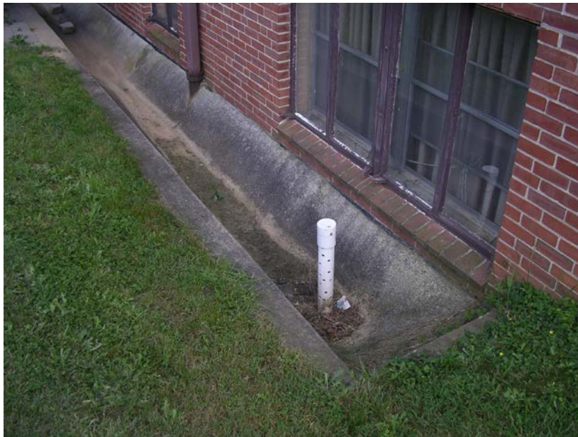
Figure 4-40: A Concrete Trough Adjacent to the Main Church Building Could be Removed and the Downspouts Redirected at ISI-A-1140.
