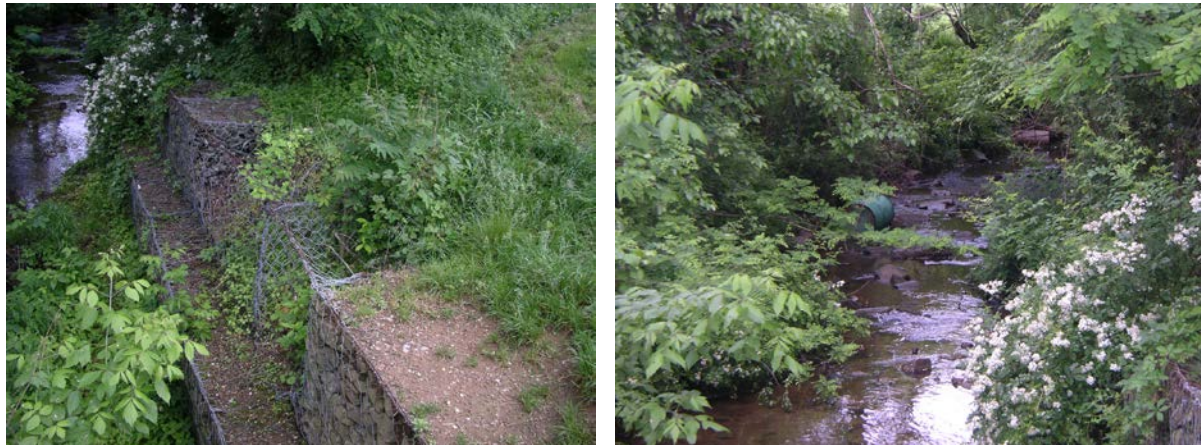
Figure 4-39: Gabion Baskets Line the Stream Banks Below the Bridge Crossing at ISI-A-1121. Some Baskets Have Failed, as Shown in the Photo on the Left. In Addition, Drums and Other Trash Litter the Stream and Offer an Excellent Opportunity for Student Involvement in a Stream Clean-up.
