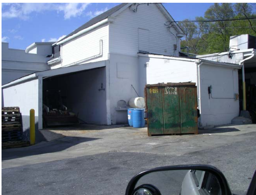
Figure 4-20: Unmarked Drums Exposed to Precipitation
