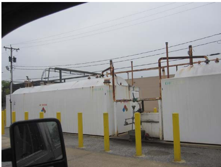
Figure 4-59: Rusting fuel lines and signs of past spills at above ground fuel storage tanks at HSI-A-1525
