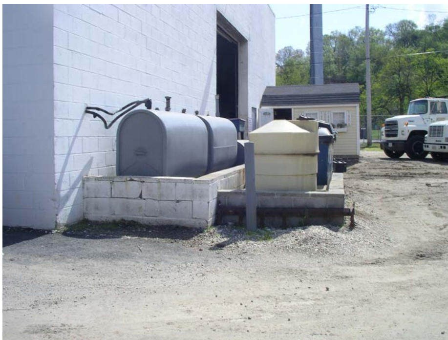
Figure 4-50: Equipment Rental Company With Cracked Containment for Oil Storage at HSI-A-1415
